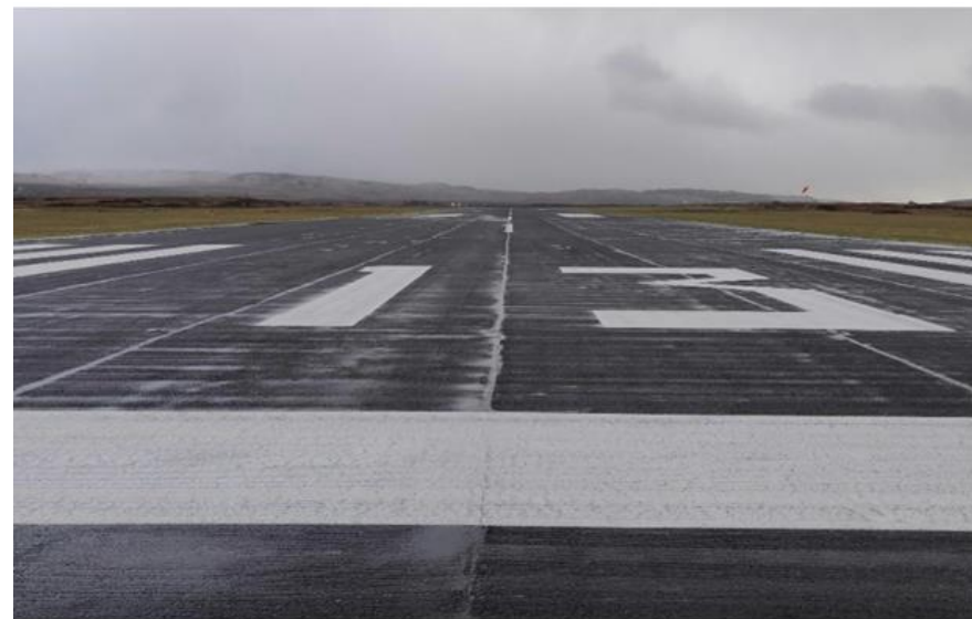
Open lane joints in the Runway 13 TDZ area
